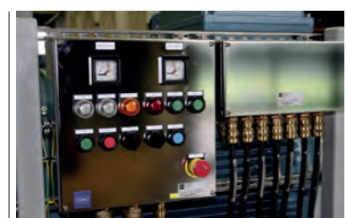
On-Off Operation by Local Control Panel
