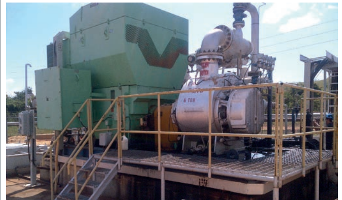
Multiphase Boosting System installed in Petrozuata Oil Field
