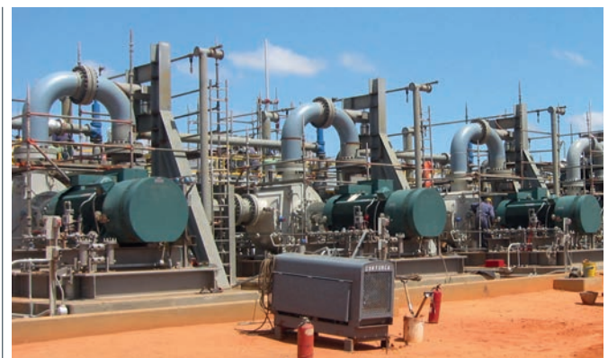
Multiphase Pump Boosting Station MW 10 Multiphase Pumps
